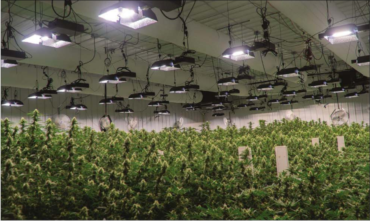
Condensation prevention, combined with antimicrobial fabrics, is one reason designers of potentially high-humidity environments, such as cannabis facilities, prefer fabric versus metal duct.
