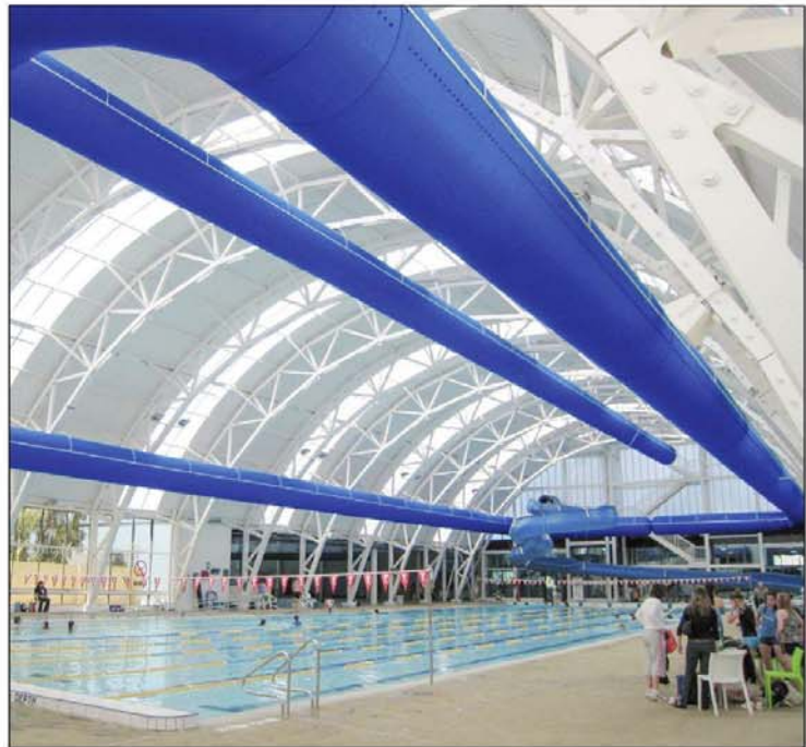
Fabric duct was chosen for this sports pool complex because natatoriums are harsh environments and have high humidity and airborne pool chemicals.
